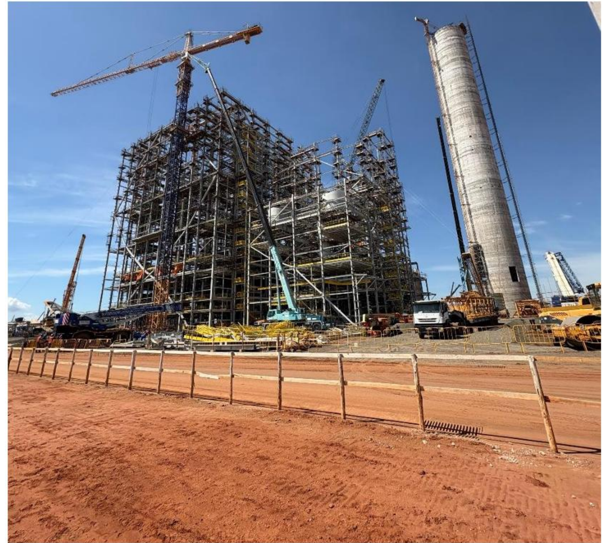
Power and recovery boilers.
